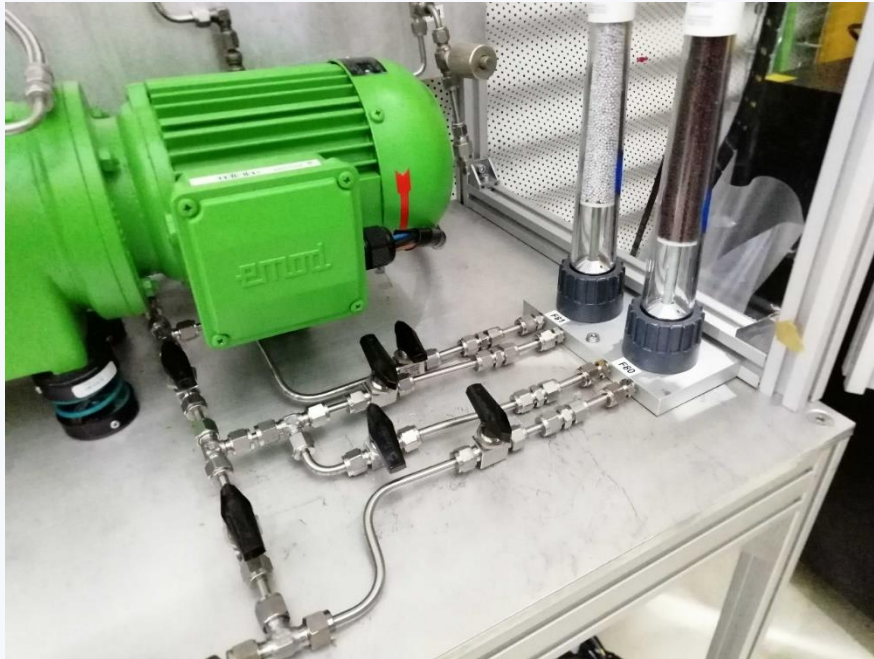
Filters in the gas system
